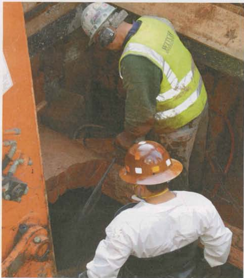
Workers cut a hole in 60-inch brick sewer built by craftsmen in 1860s. Sewer is still in excellent condition.
