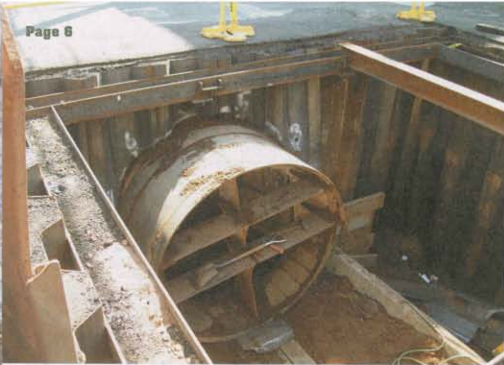
Some sections of 72-inch RCP storm water sewer, as shown in this photo, have to be jacked with only 2-½ ft. of cover.
