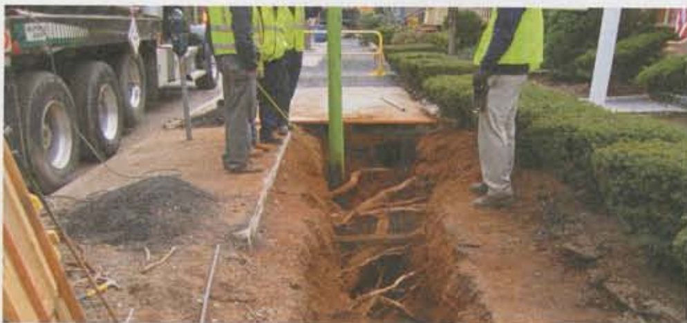
Tree roots were located using ground penetrating radar, with the information leading to the decision to jack pipe below roots to protect the trees.
