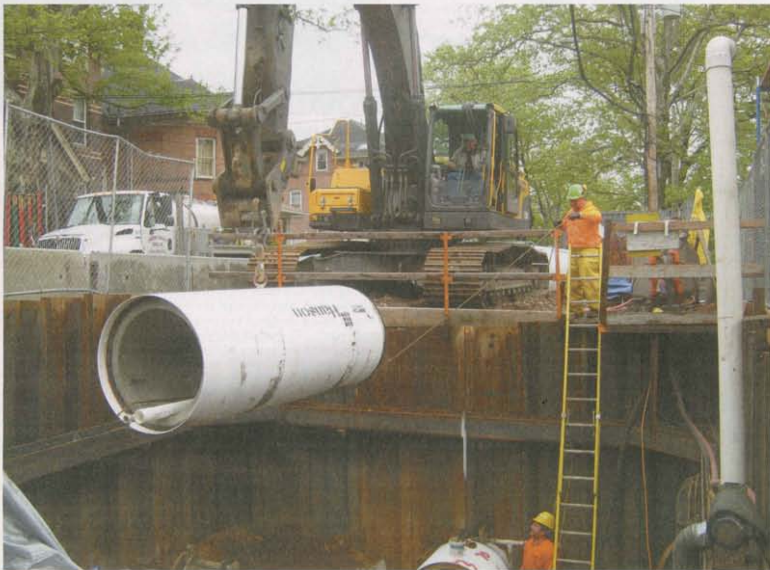
A Volvo excavator places 36-inch RCP pipe manufactured by Hanson Pipe and Precast into one of three jacking pits built for sewer separation project.
